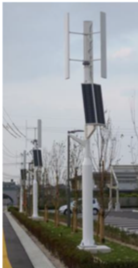
Streetlight with a small wind power generator
